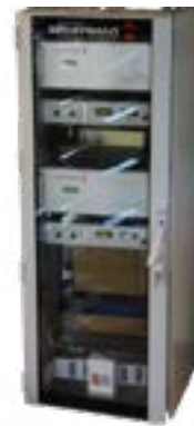
NAVTEX rack with two redundant transmitters
