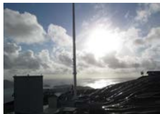
DANPHONE'S NAVTEX SYSTEM IN THE SEYCHELLES
