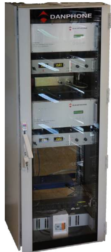
Example of MSI NAVTEX rack with two redundant transmitters.
