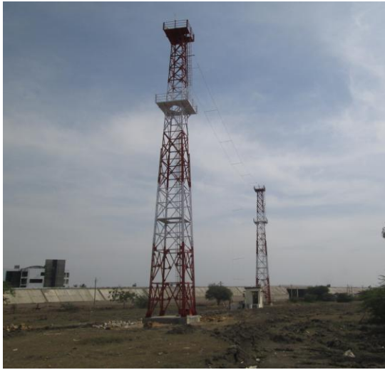
Danphone's NAVETX installation in India
